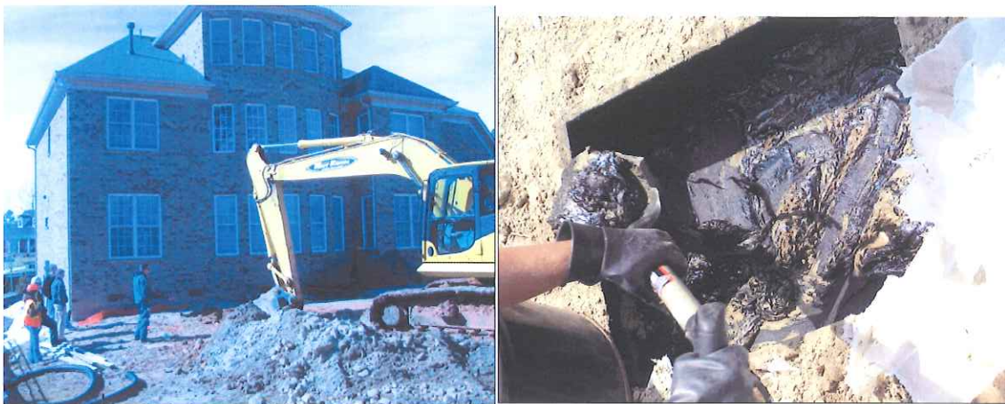
While installing an irrigation system at a home, a junction box and PVC piping were discovered. The piping came from the direction of a closed facility. The box's black sludge contained high concentrations of PCE and TCE. Air vapor samples were also taken from the crawlspace of the home and all concentrations were within acceptable range for vapor samples.
