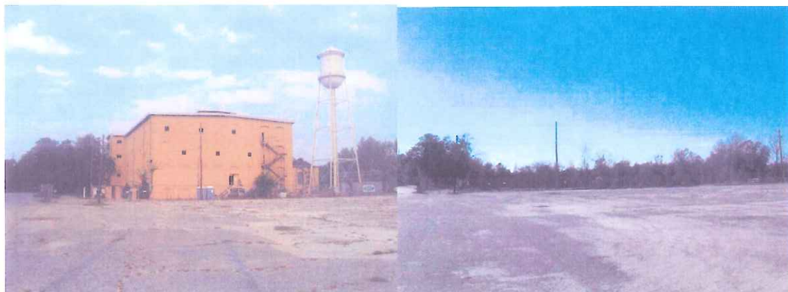
On June 25, 2008, a Responsible Party under a Voluntary Cleanup Contract began the removal of the former Nytronics Component Group, Inc.'s historic, four-story, main manufacturing building, the water tank, as well as other outlying buildings. The photo on the right was taken on November 21, 2008. The site's main contaminants of concern are PCBs and VOCs (primarily TCE). Future response activities include: the soil, the onsite sewer system, the western drainage ditch, the onsite and offsite groundwater, and Swift Creek and the associated wetlands.
